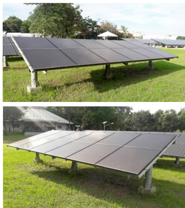
Fig. 1. 1.2 kW PV system at SGtech, Phitsanulok, Thailand.
