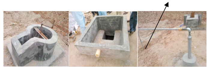
Fig. 3. Pictorial views of installed biogas plant
