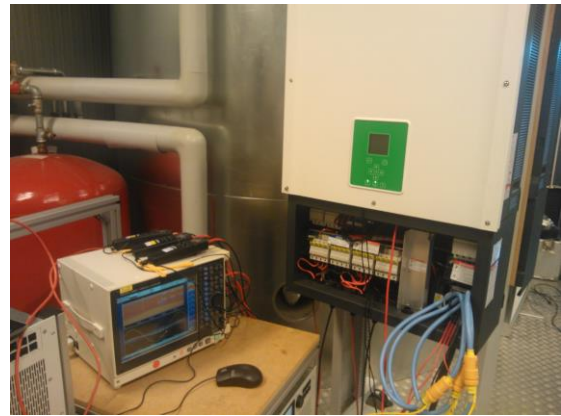
Fig. 10. Hardware test set up of PV generator with Hybrid controller
