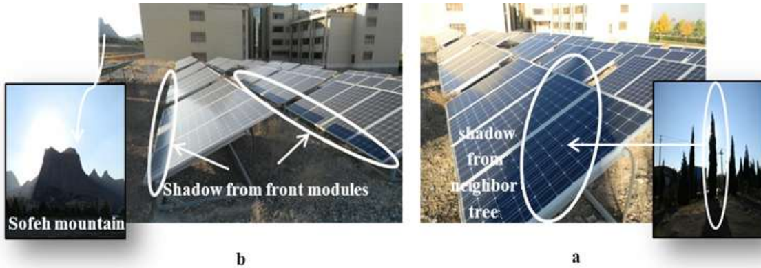
Fig. 10. Types and sources of shading on the module arrays a- morning shading b- afternoon shading
