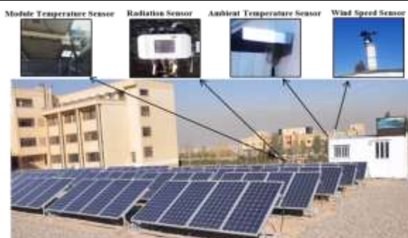
Fig. 1. 20 KW PV pilot plant installed at the University of Isfahan Iran.
