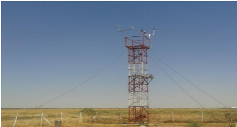
Fig. 1. Measuring mast for wind data at n'djamena airport
