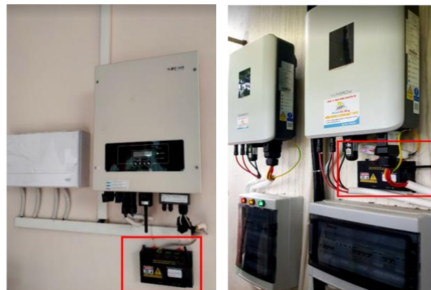
a. Inverter 1 phase b. 3 phase inverter
