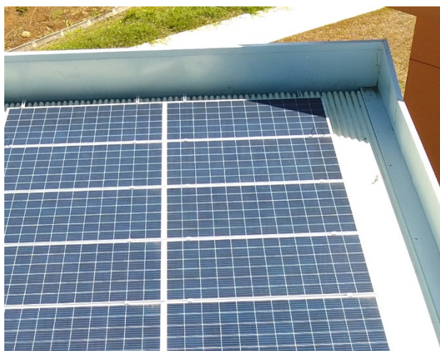
Fig. 1. Example of a solar panel with a partial shadow.
